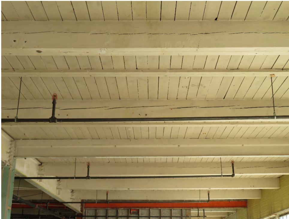
Figure 3 Multiple short, discontinuous checks near the pith that extends along the length of two adjacent timbers
